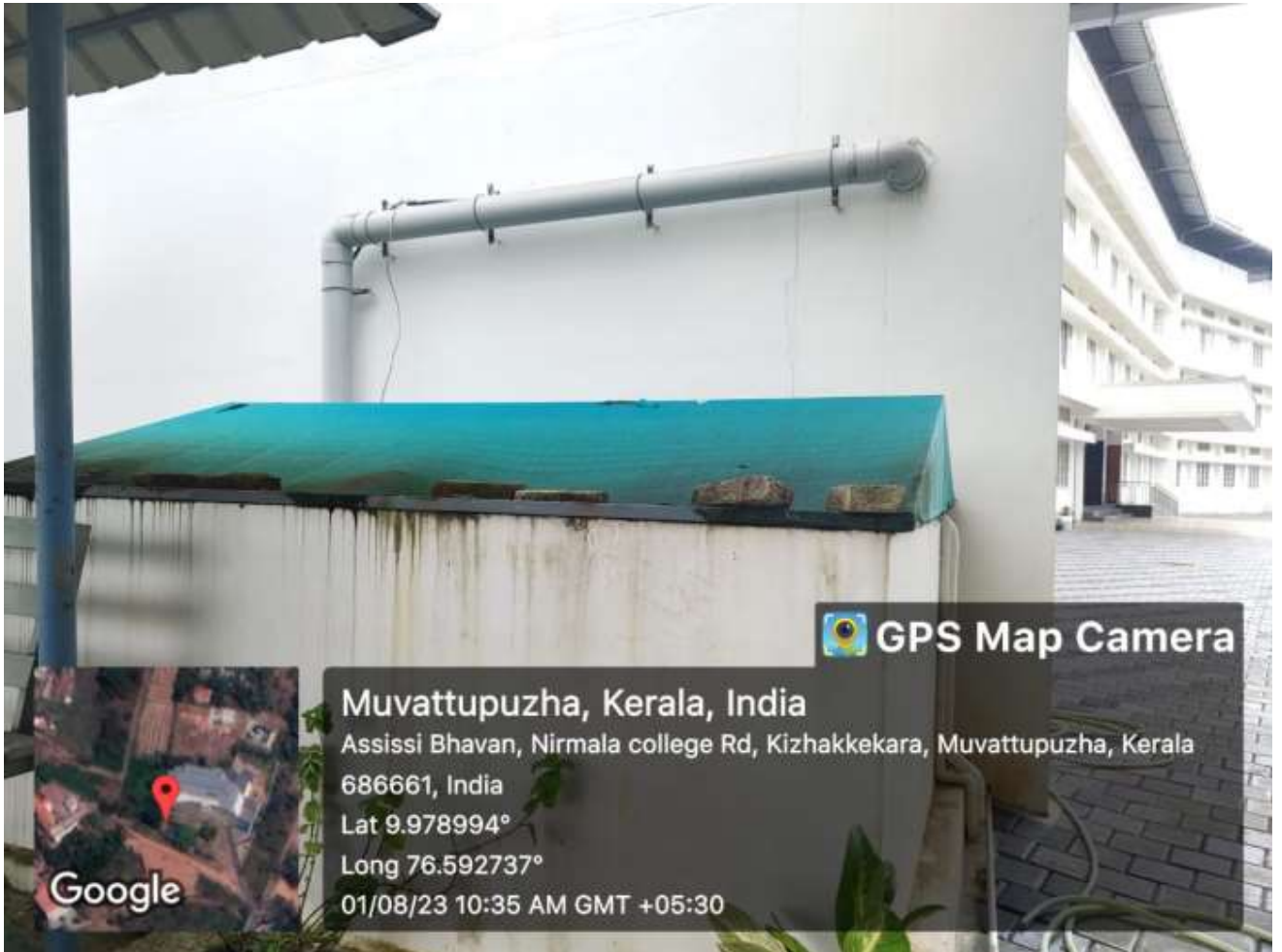
Rain water harvesting tank
